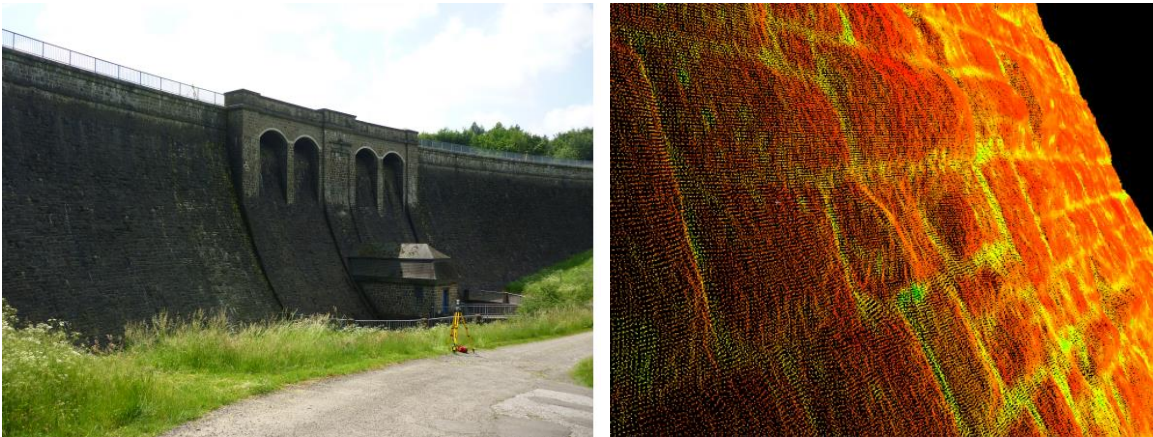
Fig. 10: Brucher water dam from the air side (left) and partial view of a corresponding laser scan (right)
