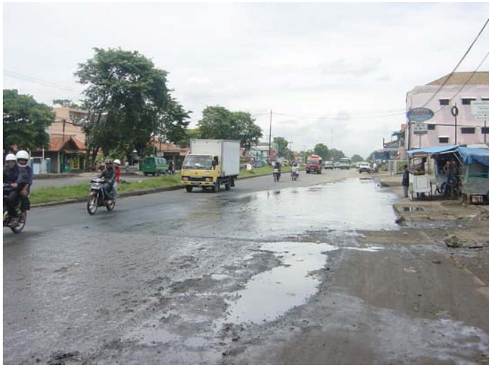
Water inundation in the road
