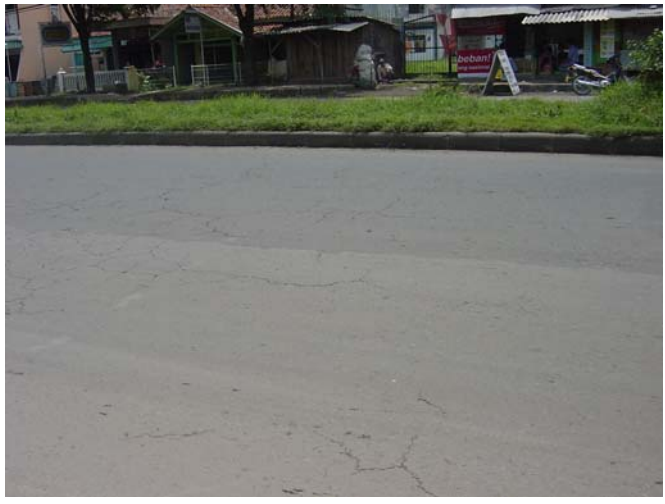
Cracking and tilting of road
